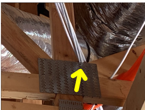
Wiring contacts sharp truss plate edge at center kitchen ceiling. As marked on the floor.
