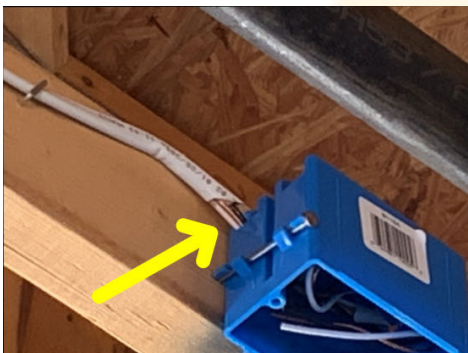
Wiring sheathing cut too short at center garage ceiling outlet box.
