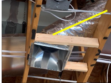
Ducting takes sharp angle, improper radius, at kitchen ceiling above the island
