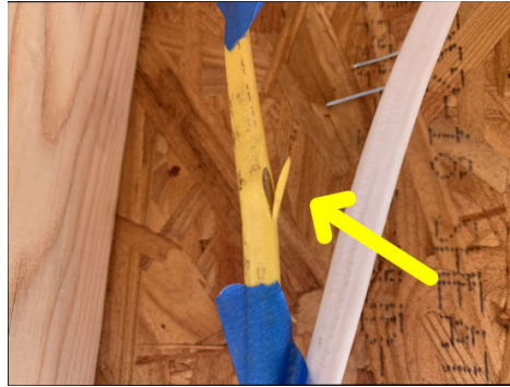
Wiring has area of damage and not secured at South East bath
