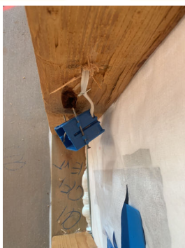
Outlet box not attached, inside east den wall
