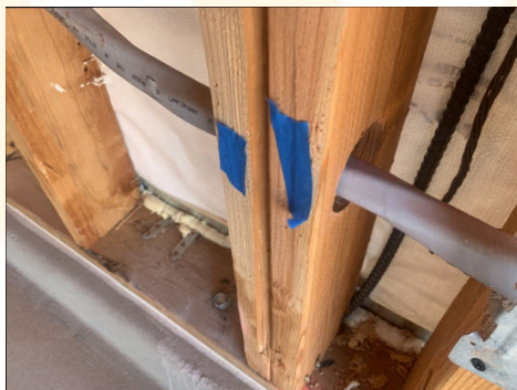
A nail plate is needed to protect the wiring that is closer than 1 1/4" from the face of the stud. Noted at: West garage wall below electrical panel at several areas,
