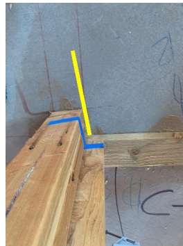
Walls are not square at . Walls should be perpendicular within 1/4" in 10'. Noted at: master water closet entry, Entry to bedroom number three,
