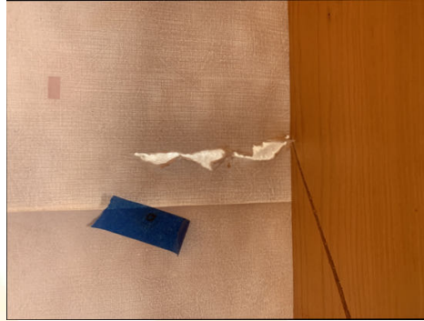
Stucco paper damaged at: West garage wall
